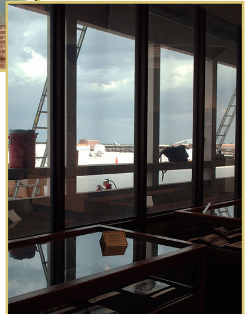
View of roofers working on the 1984 4 th floor roof (as seen from the 1968 5 th floor windows).
